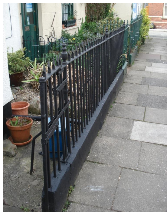
Fig.38 A typical set of cast iron railings to small front gardens, these examples may date to the late 18 th century
