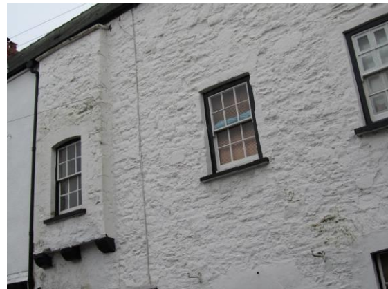
Fig.102 Part of the Great House of Roger Williams, in Old Market Street, illustrating some of the subtlety of the construction, which raises questions regarding the age of its construction.
