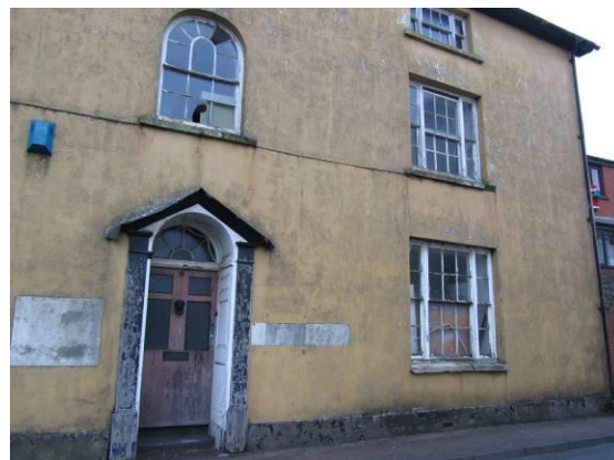
Fig.124 No.10 Old Market Street- a fine Georgian town house in very poor condition.
