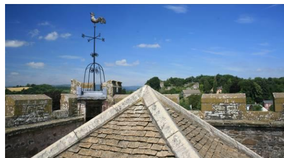
Fig.164 Stone slate is used on a collection of buildings, notably the parish church
