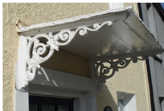
Fig.37 Cast iron decorative brackets to doorhoods – a distinctive pattern which is repeated on a number of notable buildings
