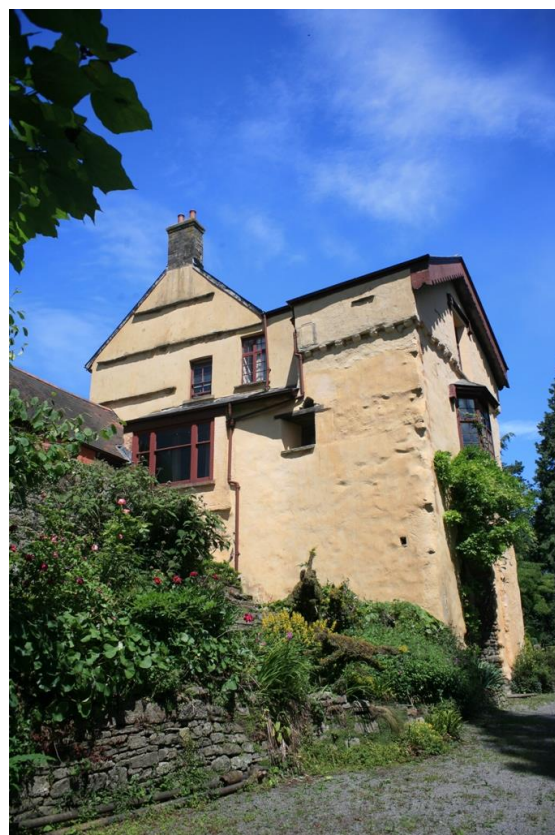
Fig.62 The Gatehouse to Usk Castle is lime rendered and has an applied coloured limewash giving the building a very distinctive and unusual appearance, but is possibly based on historic precedent
