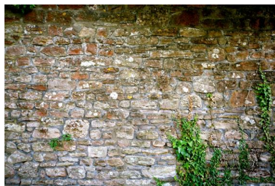
Fig.60 Typical colouration to the rubblestone walls
