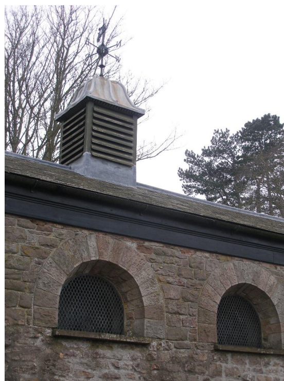
Fig.52 Detail of the Stables, showing its louvered cupola and boldly expressed semi-circular high level windows
