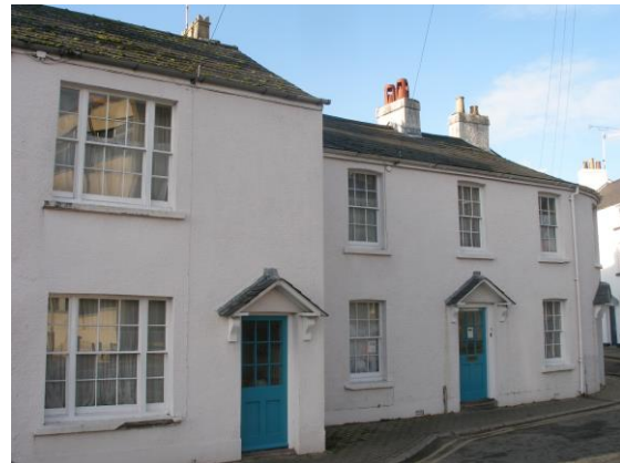
Fig.181 An attractive range of cottages in Chippenhamgate Street, some with handsome tripartite sash windows
