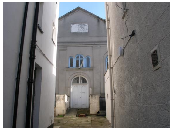
Fig.144 A glimpse of a former non-conformist chapel behind the frontages of Monnow Street. Its classical mouldings are somewhat eroded
