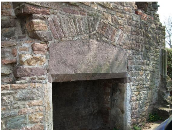
Fig.85 Coursed rubblestone seen on the ruins in the grounds of the Procurator's House
