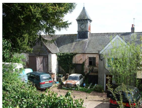
Fig.51 Court Farm. This range with its eye catching clock tower is unfortunately in a poor state of repair
