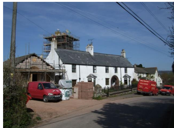
Figure 12 The Old Vicarage, one of a number of larger buildings within the village
