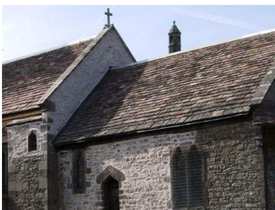
Figure 32 Stone slates are a feature of St John's church. These are traditionally laid in diminishing courses which gives a very attractive highly textured roof finish
