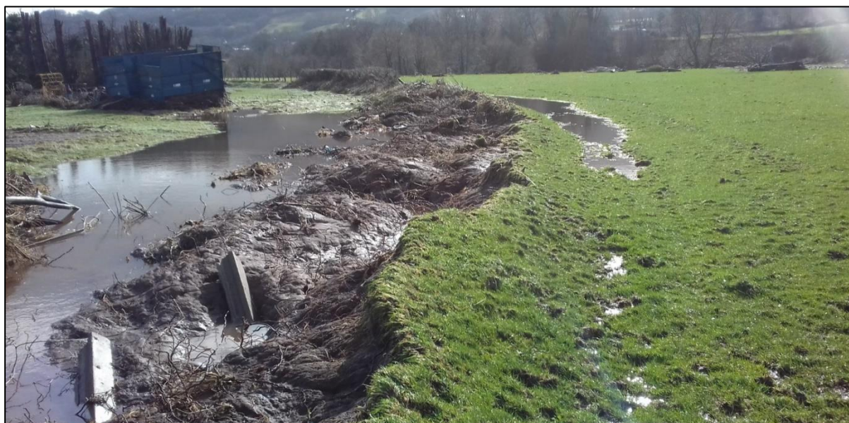
Photo 3: The southern breach in the flood embankment.
