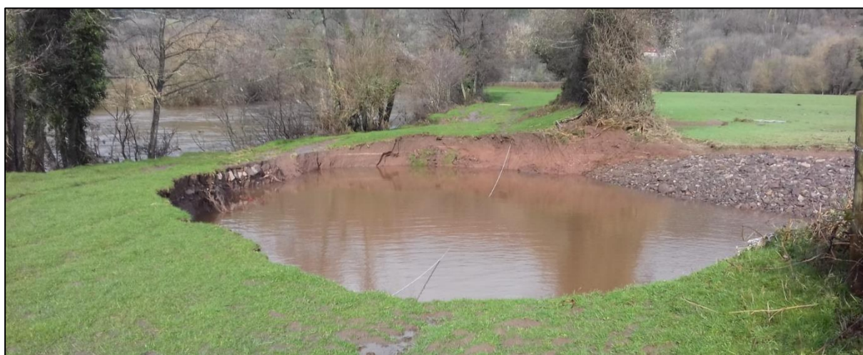
Photo 1: The crater in the flood embankment.
