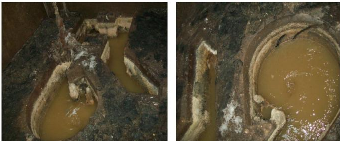
Figure 5 – Undy Main PS wet well and incoming sewer
